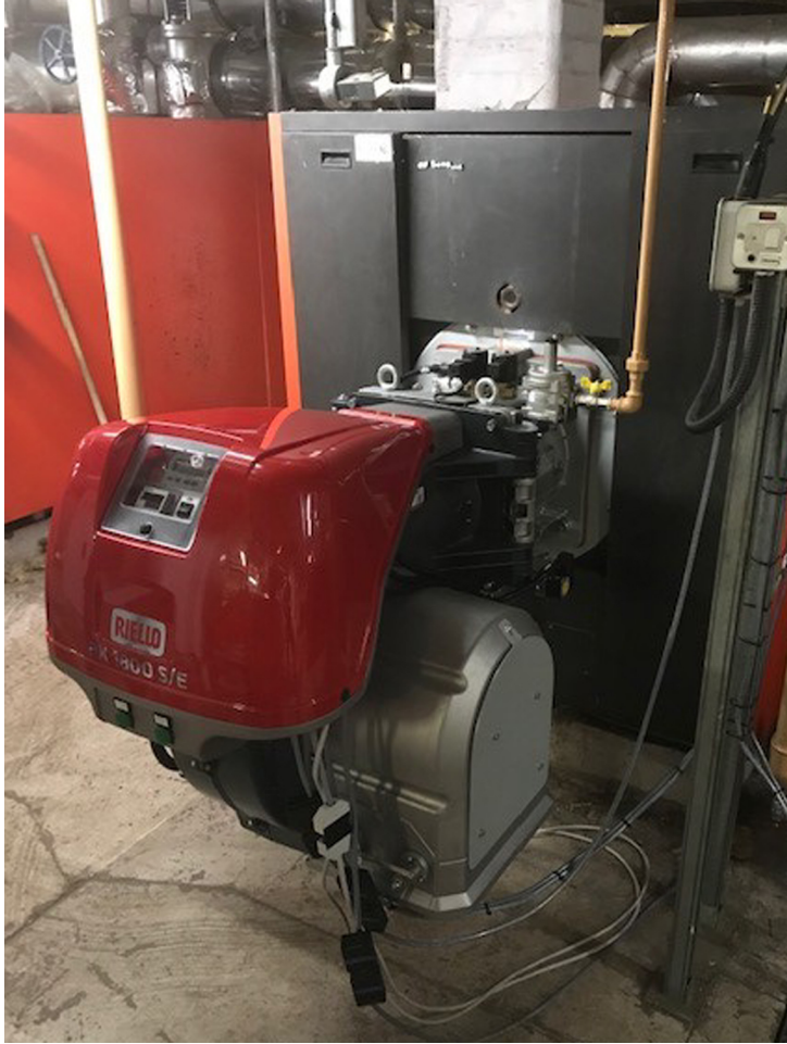
Caption: A Riello RX1800 1.8MW burner
